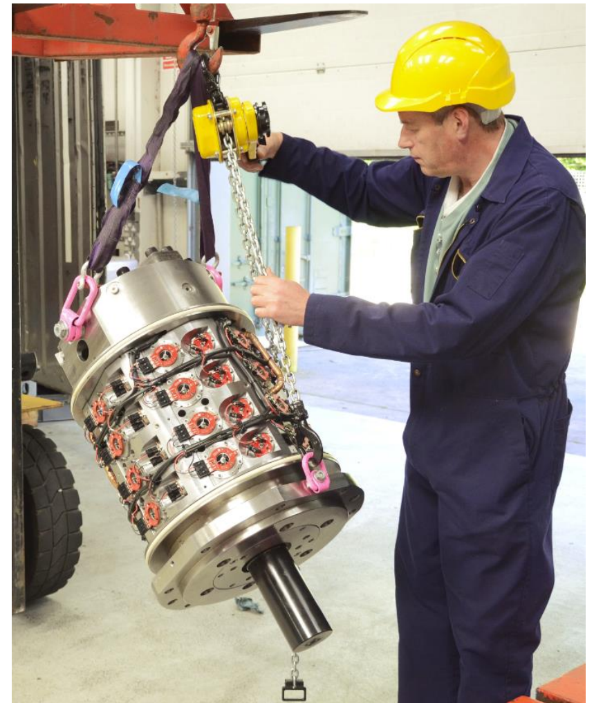
David Cruikshank fitting the 800kW DDM (with cover removed) to the generator.
